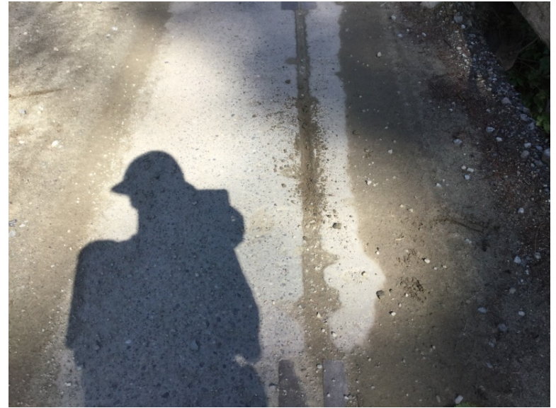
Joint sealant nonexistent
