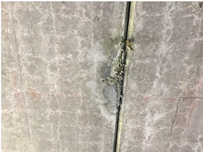
Spall under slab 4 at center
